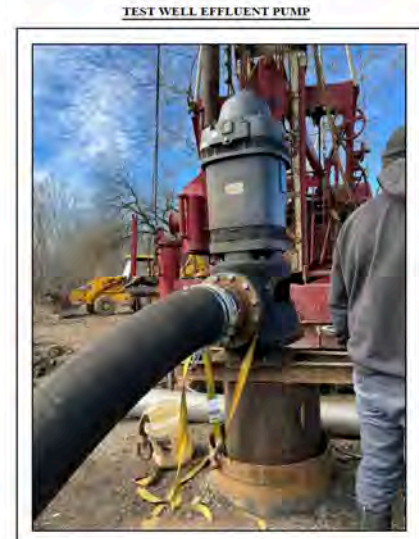
Contractor to ensure all well effluent is captured and discharged directly to Raccoon Creek. Contractor to minimize disturbance to surrounding area. Disturbed areas shall be seeded and mulched per ODOT CMS 659.
